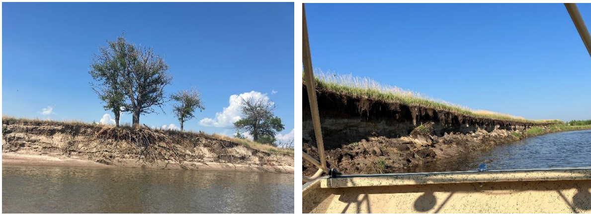
Figure 2.4. Field photos from July, 2024 depicting high eroding banks in the J2 Return Channel.
