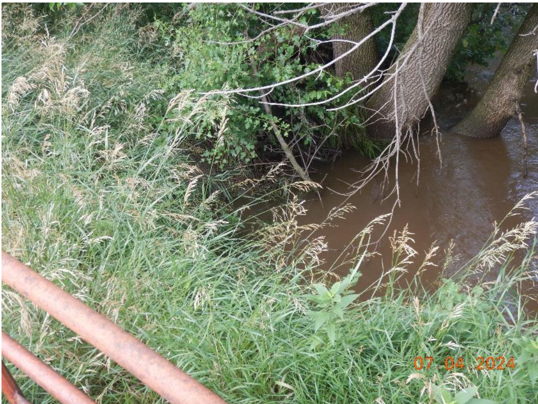
Photograph 12. Potential erosion/scour upstream of County Road 430 culvert.
