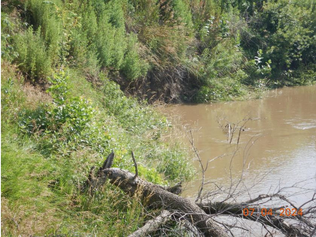
Photograph 19. Potential erosion/scour downstream of County Road 432 bridge.
