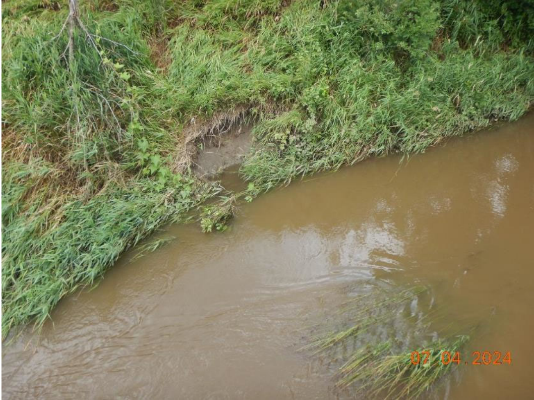
Photograph 7. Potential scour/erosion upstream of County Road 429 bridge.
