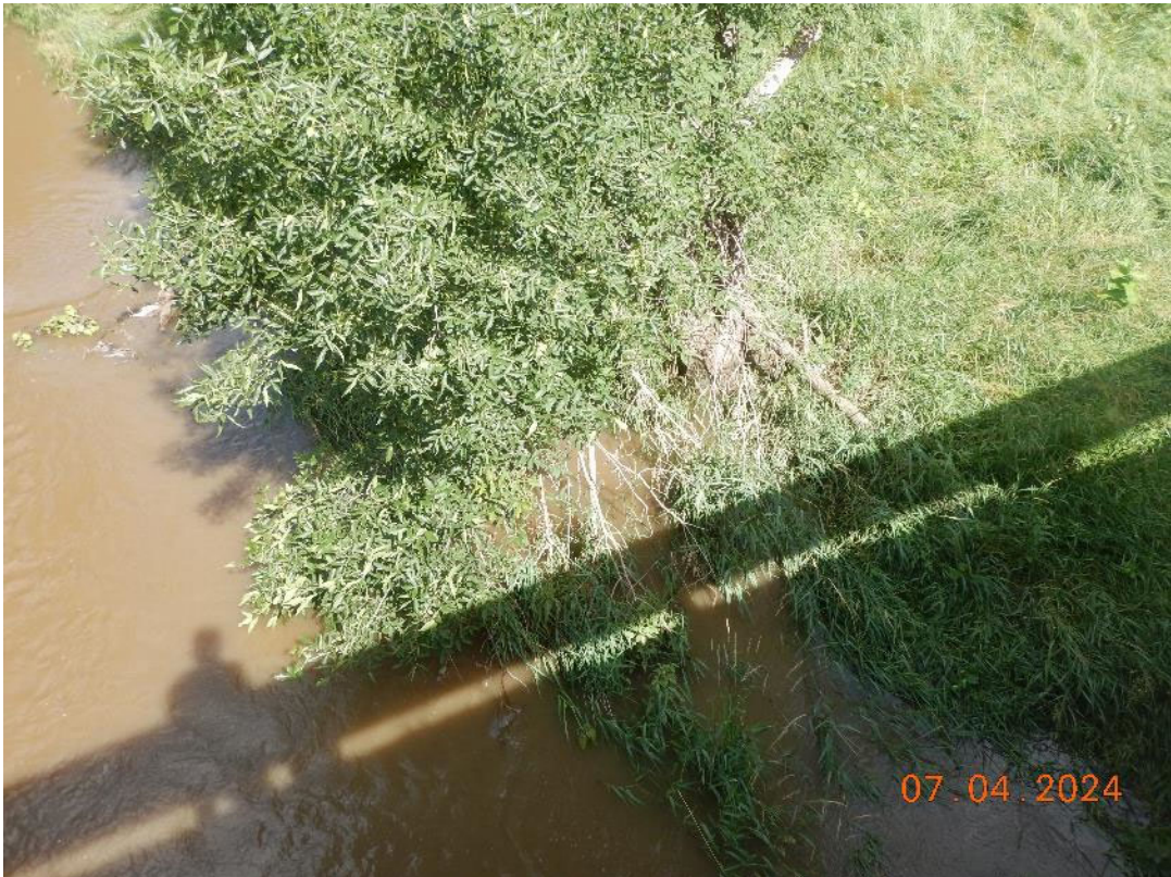
Photograph 22. Potential erosion/scour upstream of County Road 433 bridge.
