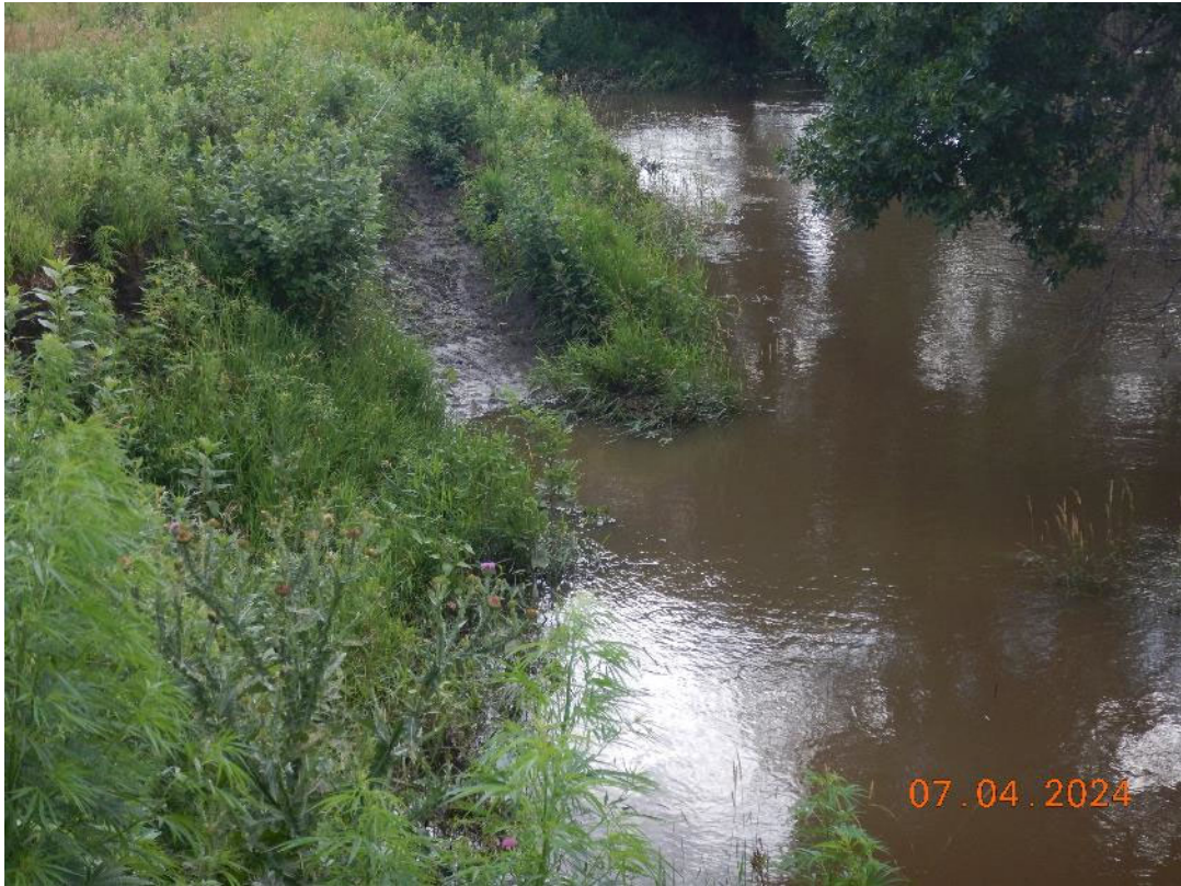
Photograph 15. Potential erosion/scour upstream of County Road 430 culvert.
