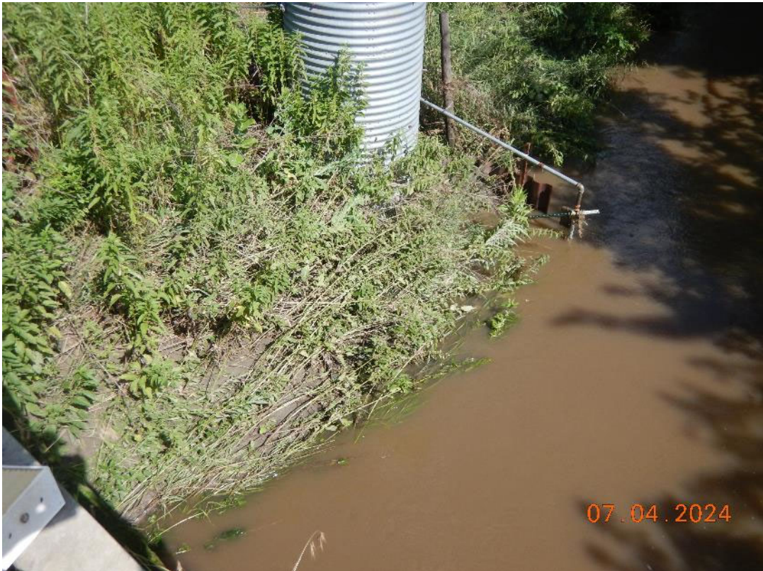
Photograph 28. Potential erosion/scour near stream gage downstream of County Road 746 bridge.
