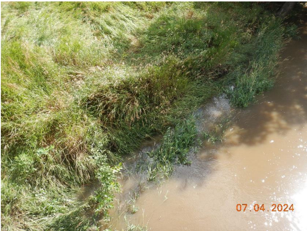
Photograph 24. Potential erosion/scour downstream of County Road 433 bridge.
